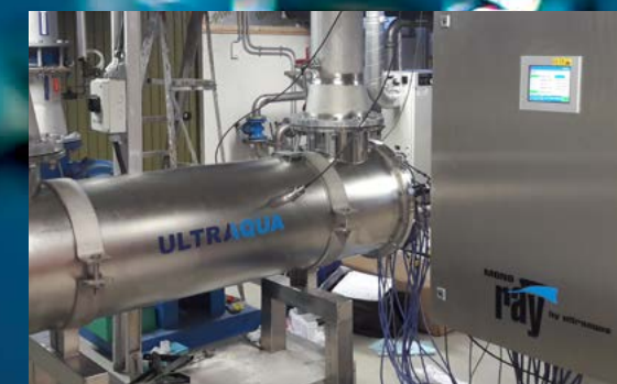
DRINKING WATER - FINLAND Disinfection of drinking water - ÖNORM validated
